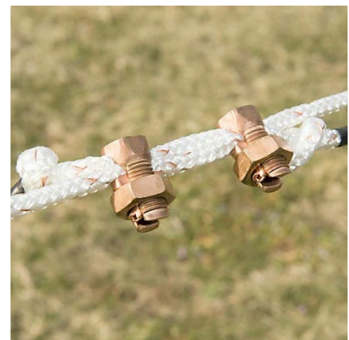
Figure 11 Split bolts used to splice Dacron line. Note the use of knots to backstop the connection.
