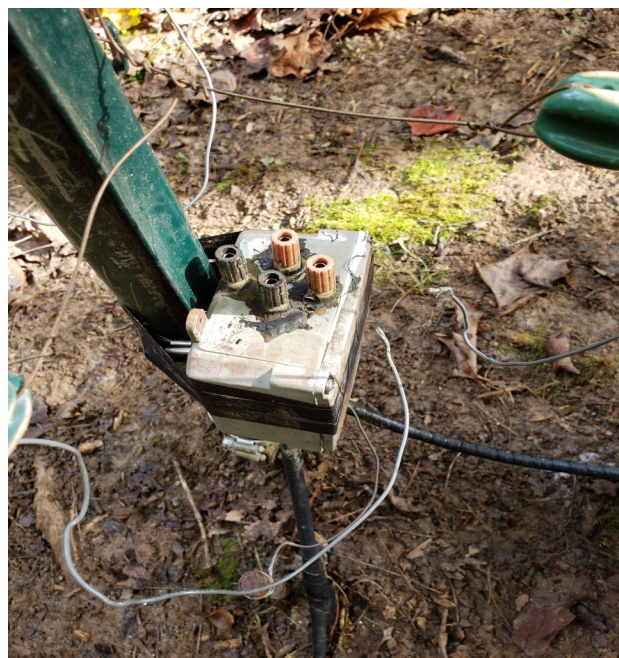
Figure 3. N4GG's K9AY Loop outdoor termination box with the antenna wires disconnected.
