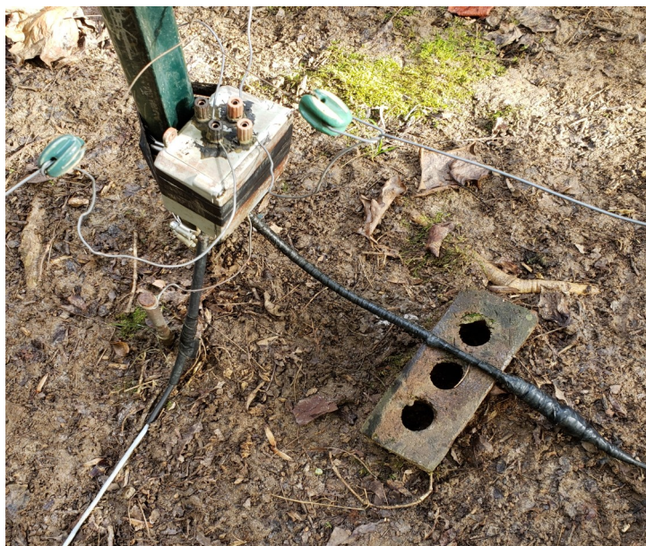
Figure 2. N4GG's K9AY Loop outdoor termination box.
