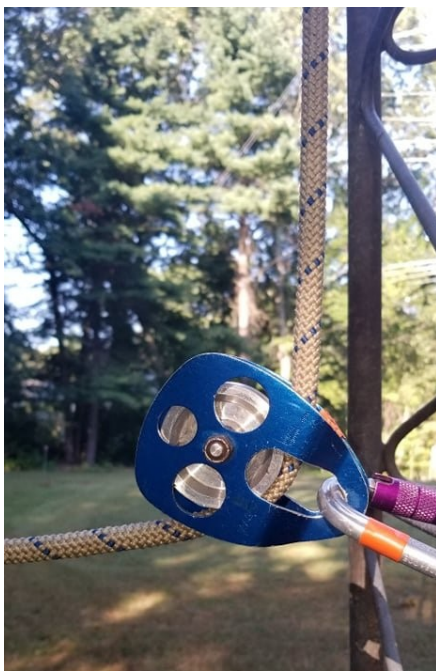
Figure 2. Use of a shackle and pulley to perform a 90 degree bend at the tower base. Courtesy of K1IR. This is a best practice.
